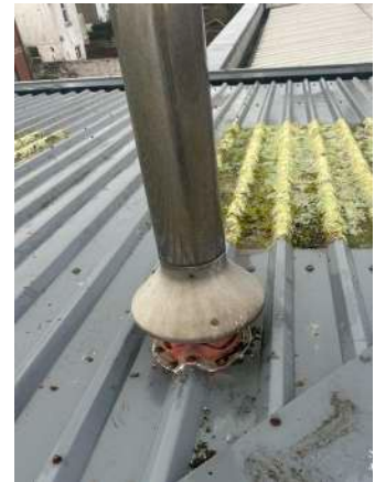
Before and After, Flue
